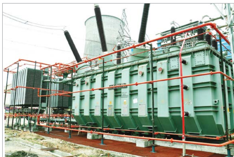
India's first 400 kV Phase Shifting Transformer
