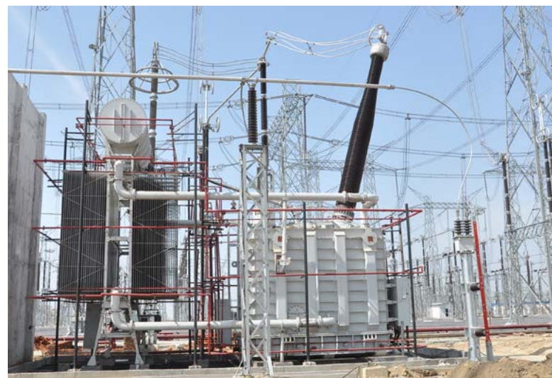
India's first 400 kV Controlled Shunt Reactor at Itarsi Substation
