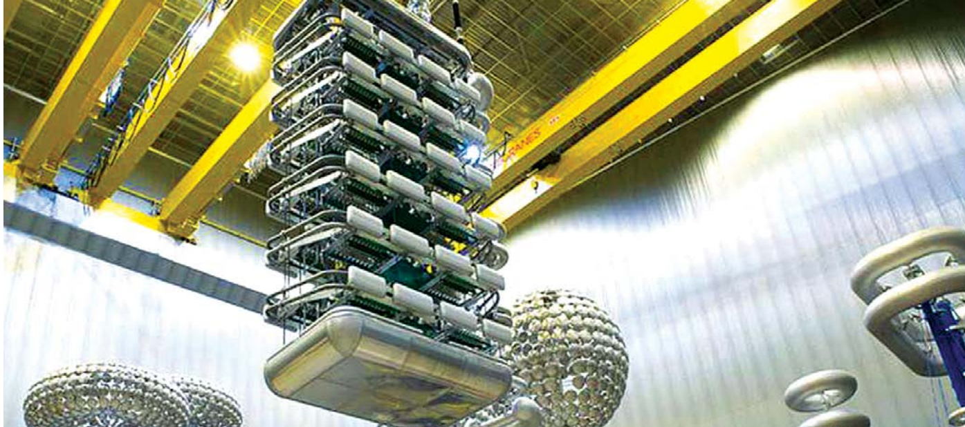
Thyristor Valves for Raigarh - Pugalur HVDC project
