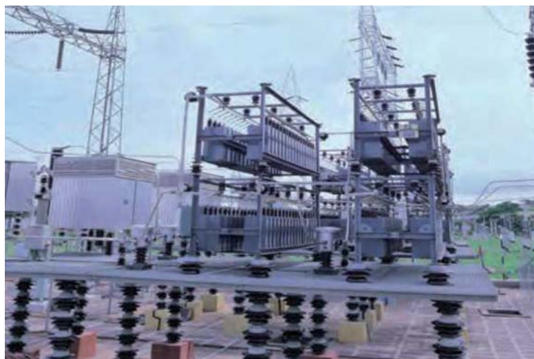
Fixed Series Compensation Scheme at Ballabgarh, India
