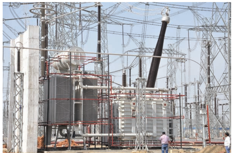
80 MVAR, 765 kV Shunt Reactor at Greater Noida Substation
