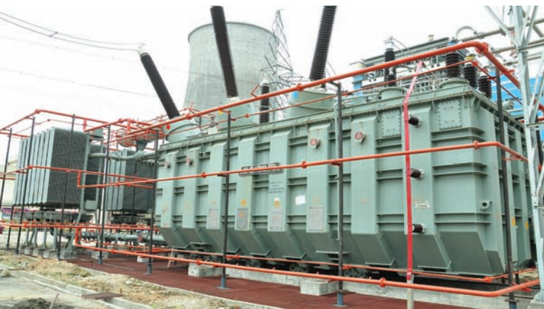
India's first 400 kV Phase Shifting Transformer at Kothagudem
