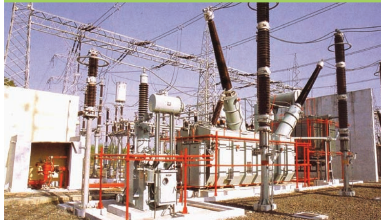
India's first 400 kV Controlled Shunt Reactor at Itarsi Substation
