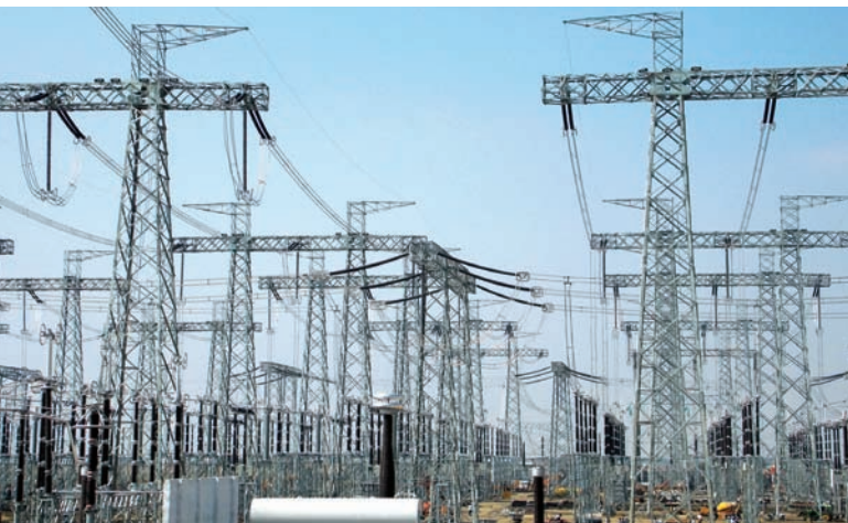
765 kV Substation at Raichur
