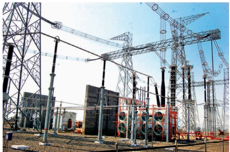
India's first 1200 kV Transformer at Bina Test Station
