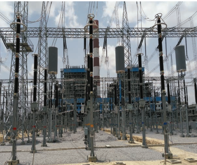
400 kV Switchyard at 2x800 MW Yeramarus TPS
