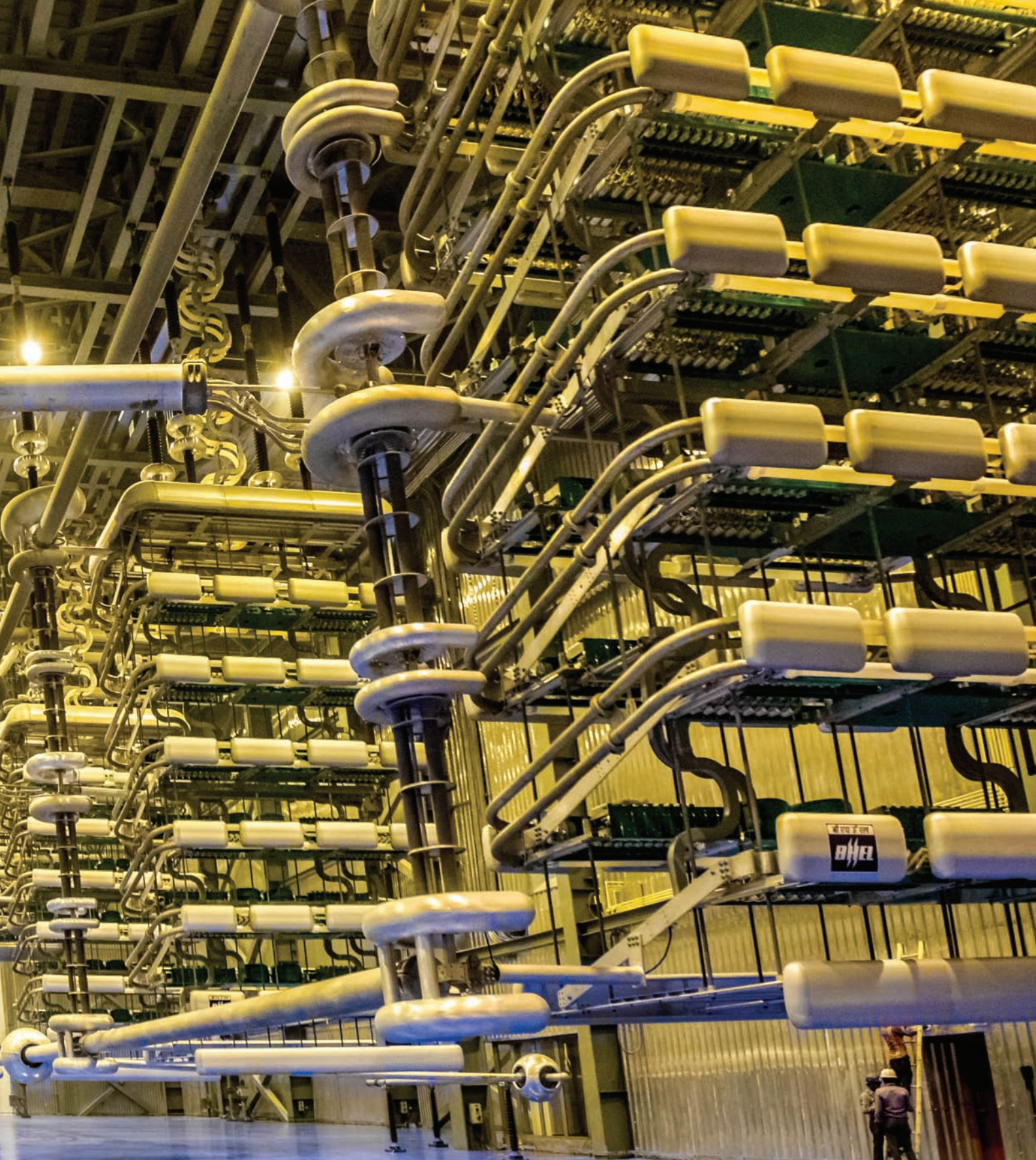
Valve hall at Agra converter station for \pm 800 kV, 6000 MW North-East Agra HVDC project
