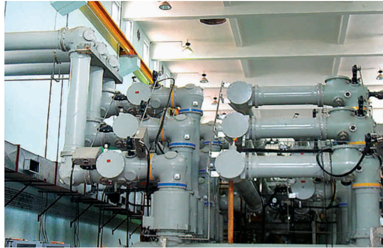
400 kV GIS Switchyard at North Chennai TPS
