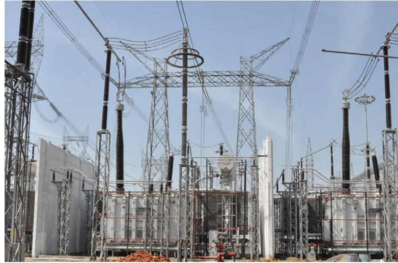
500 MVA, 765/400 kV Auto Transformer at Greater Noida Substation
